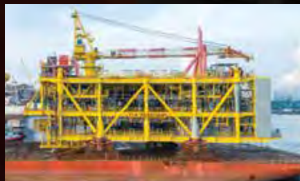
Well Head Fixed Platform Topside
