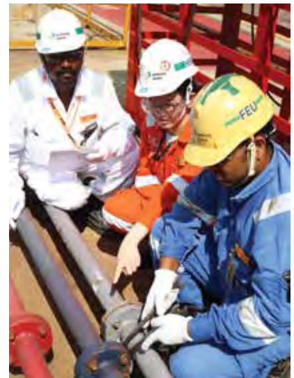
Regular leak checks are conducted on utility pipelines to eliminate wastage of resources
