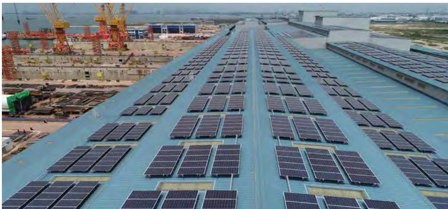
Tuas Boulevard Yard boasts Southeast Asia's largest single solar rooftop in a shipyard
