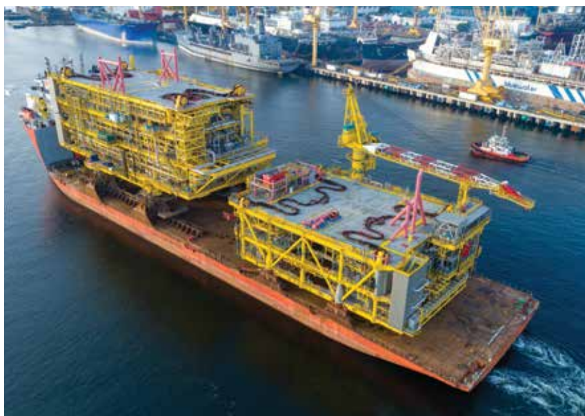
Sembcorp Marine delivered offshore production platform modules, topsides and ancillary facilities to TOTAL for the Culzean field development
